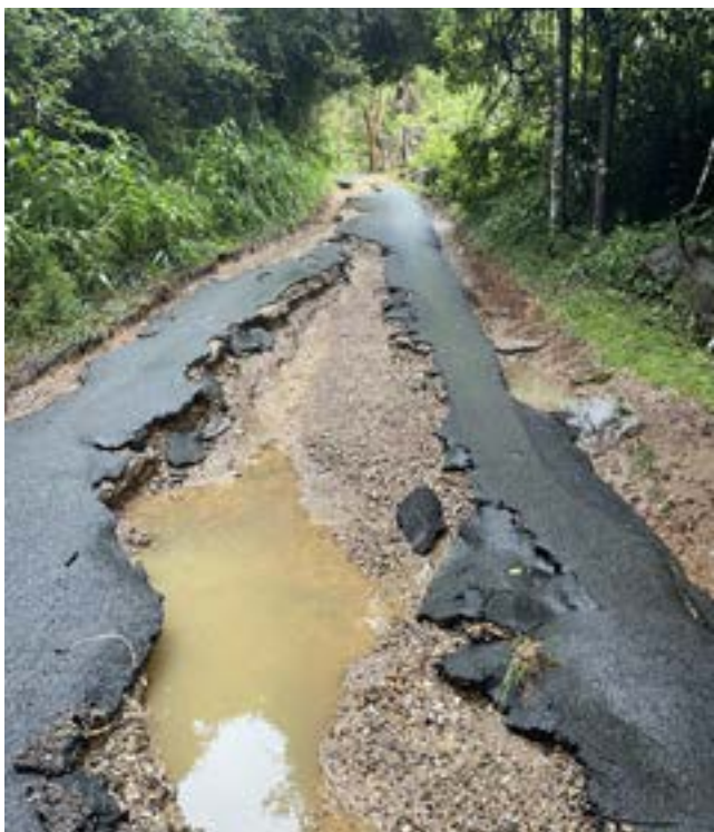
Receding flood waters exposed extensive damage to large sections of local roads.
