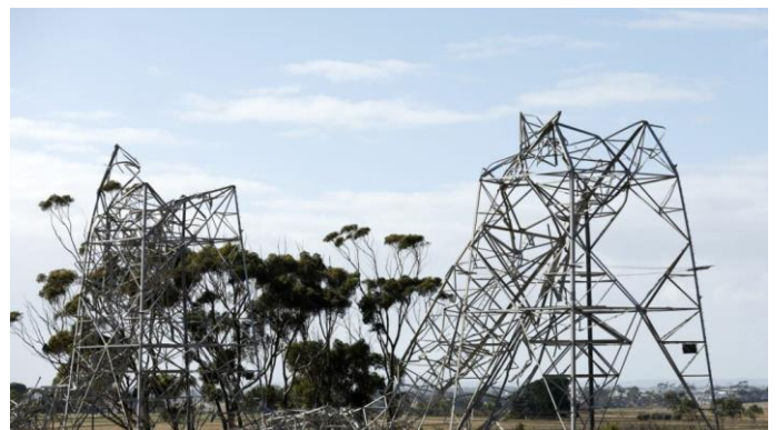
Damaged transmission towers at Anakie in Melbourne, Wednesday, February 14, 2024. Photo: AAP/Con Chronis
